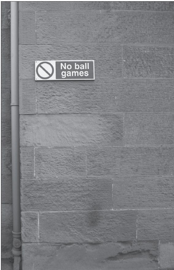
Fig. 5. Accelerated decay in original masonry with removal of the horizontal broached work effected by excess water run-off from the plastic sign. (Photo A. A. McMillan.)
