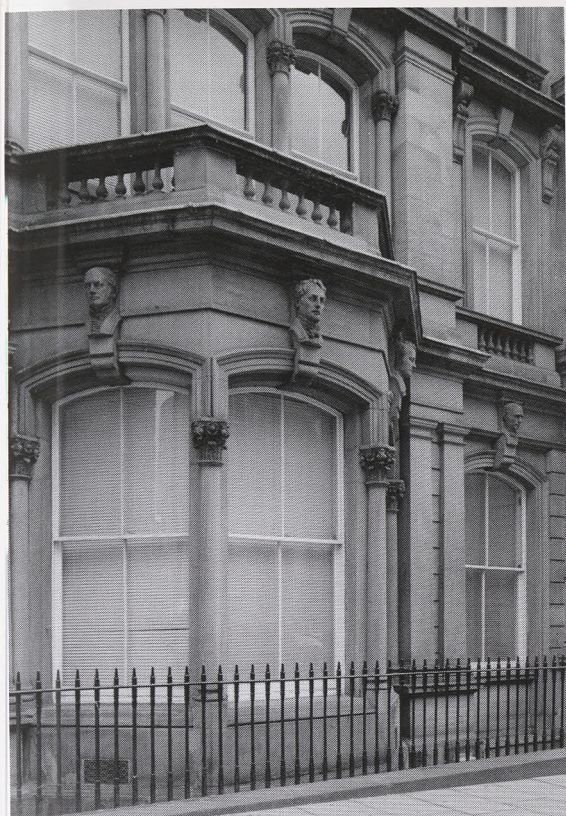
Fig. 9. The former Phrenological Museum in Chambers Street, July 2001. While the Museum's original bay window is seen to the left of the photograph, the original entrance doorway, on the right, has been converted into another window. Note the sculpted heads on the keystones. (Photograph courtesy of Joe Rock.)
