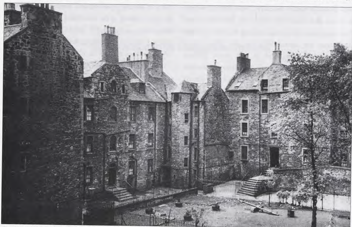
Fig. 2. North front of Chessels Building, including west wing and southern block of West Tenement, before refurbishment. (Hurd Rolland Partnership.)
